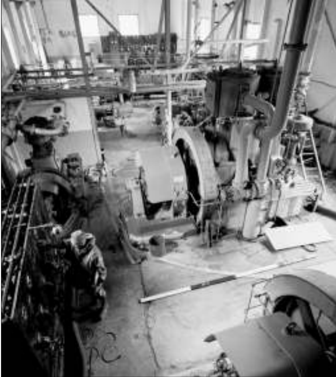
The Bergen generators at Stromness.. The control panel is at left. Dag Naevestad, Industrial Archaeology at South Georgia (NARE 89/90)
