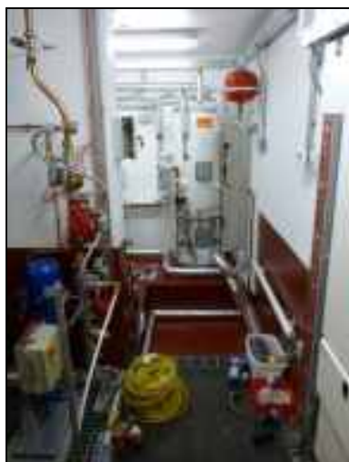
Part of the new boiler room. There is an electric boiler using power from the hydro-generator below Gull Lake and a diesel boiler as standby. The room also houses pumps for sewage and the fire sprinkler system.
