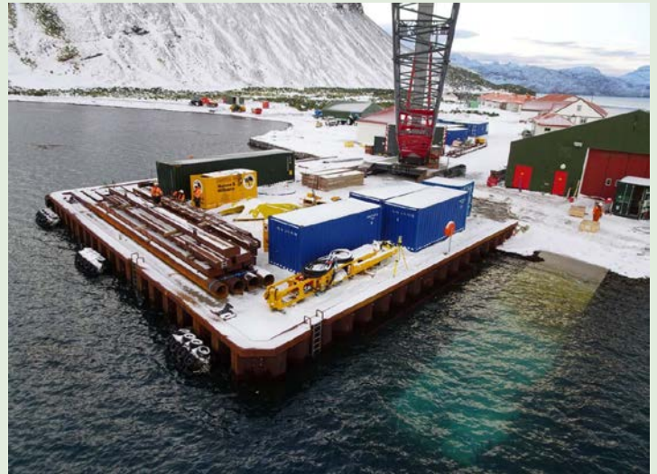
The new jetty at KEP with the new slipway visible on the right.
